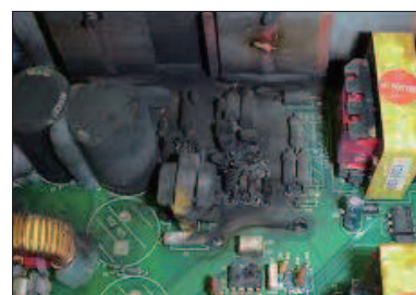
Damage to fuse
